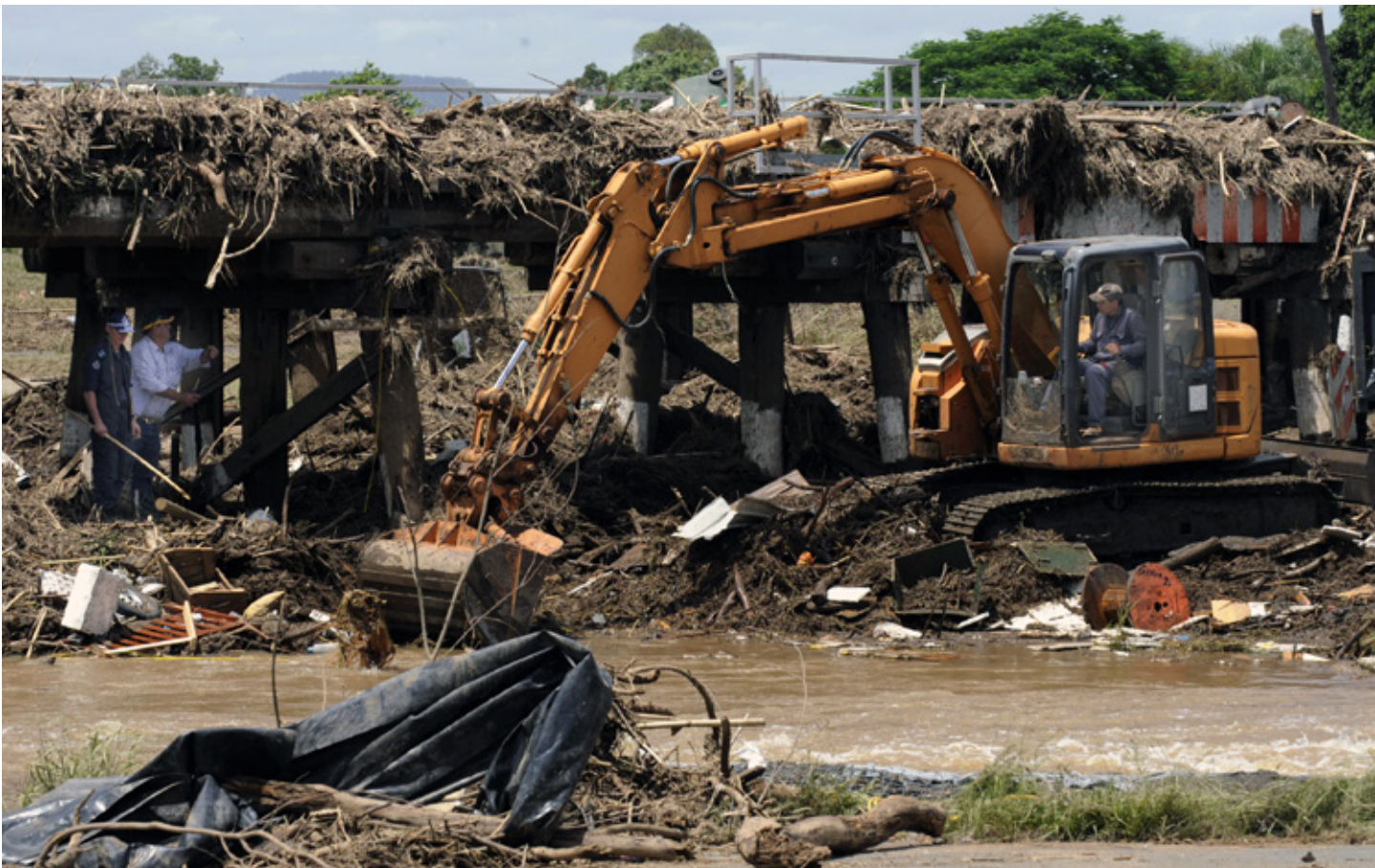
Earth moving equipment was brought in to clear debris from the railway bridge after floodwaters receded in Grantham, west of Brisbane in Queensland. (Jon Hargest/Newspix)
