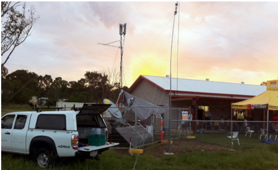
A community outpost staged at the local pub. The community of Murphy's Creek was isolated from all communications during the disaster so Optus deployed a SatCat mobile base station to provide communications and support for a number of weeks. (Optus)
