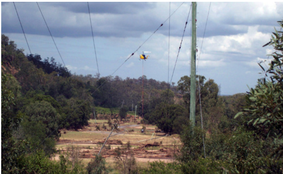
Optus engaged the resources of a Helicopter Charter company to transport a 5km drum of cable to repair and reconnect the Optus Network as soon as the water receded. (Optus)
