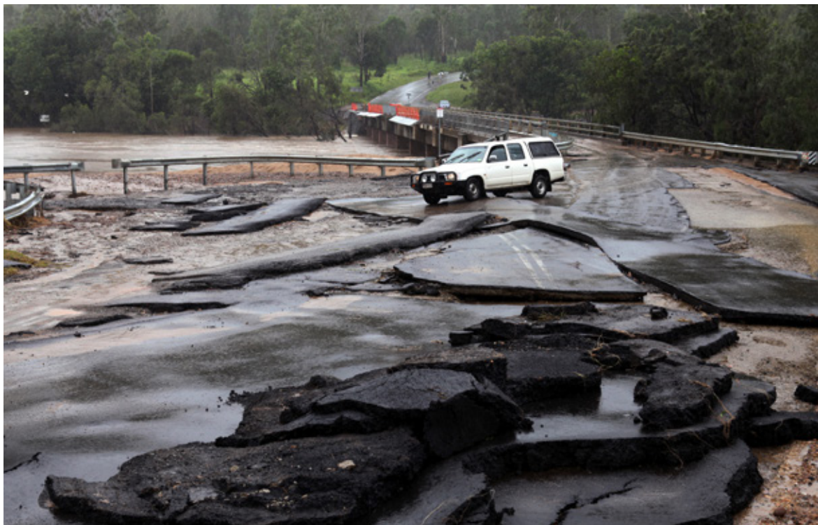
The Kholo Road and bridge over the Brisbane River, was seriously damaged by floodwaters, December 2010, Queensland. (Tim Marsden / Newspix)
