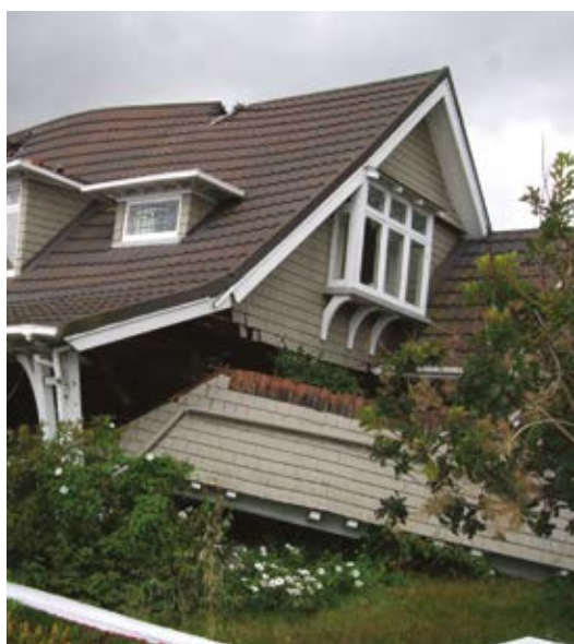
Christchurch, New Zealand: Following three major earthquakes since September 2010, geotechnical experts divided Christchurch into four zones – red, orange, green and white. Residents in the worst-affected red zone received a formal offer from Government to buy their homes.
